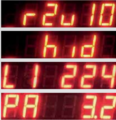
Figure 8. Panel Main Operating Screen
