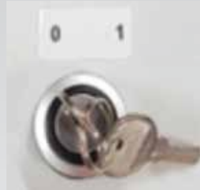
Figure 7. On-Off Button of Diesel Control Panel
